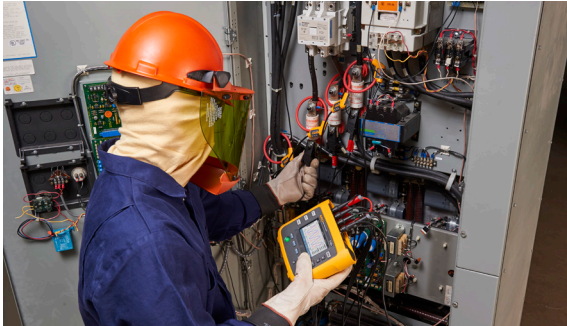
Using a Fluke 1738 Advanced Power Energy Logger to perform an energy study on a mechanical system
